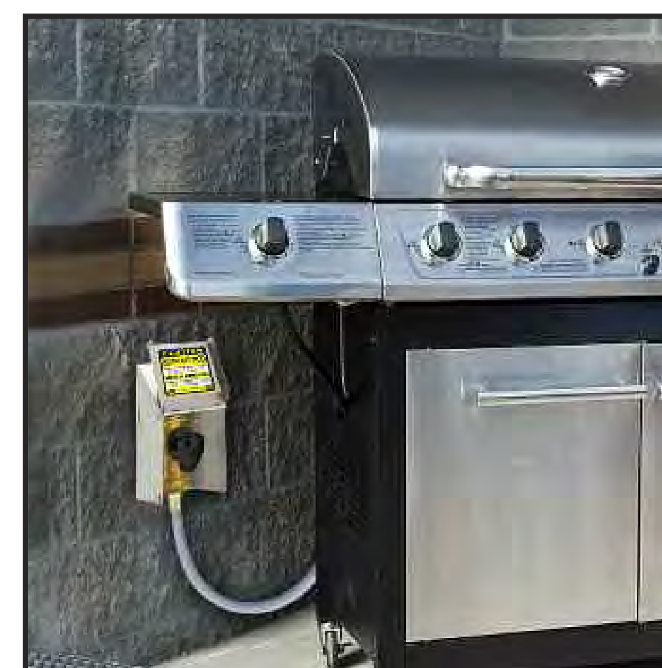
Hose Assembly Length Restrictions May Apply: Check with Local Jurisdictions
