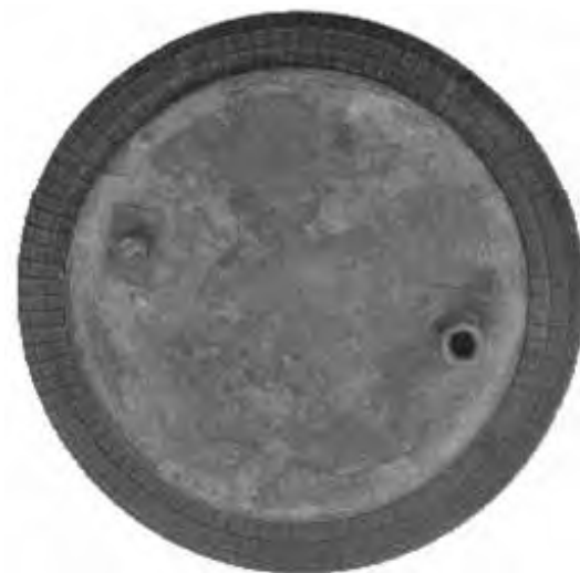
CORROSION AND IMPACTS
